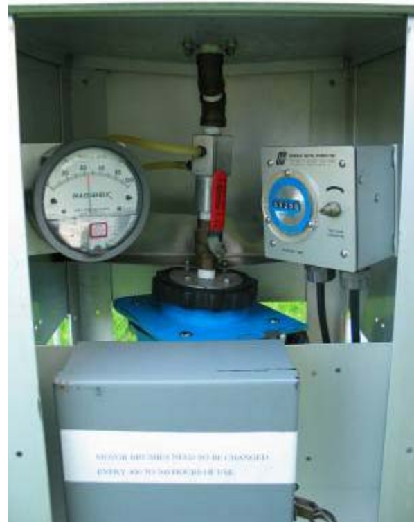
Inside Front Compartment
